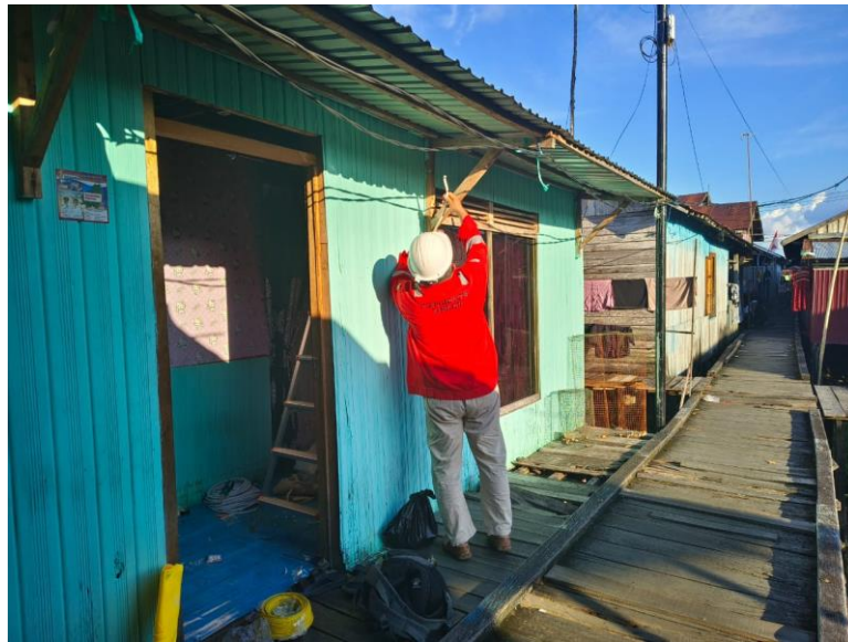
Figure 2. Electricity Installation in Bukit Tunggul Subdistrict
